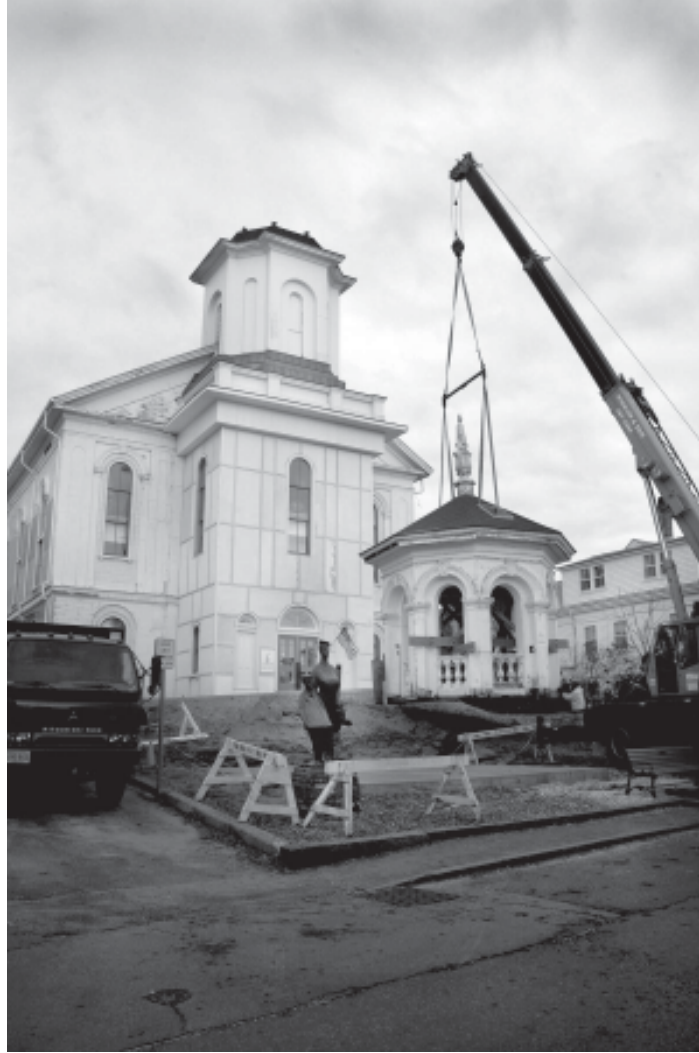
Crane moves Library belfry to temporary resting place while the structure awaits renovation and placement atop the building once funding goals are achieved.
