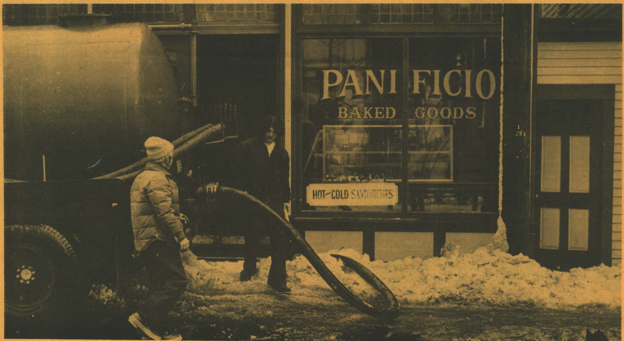
Pumping out Cicero's Trattoria
