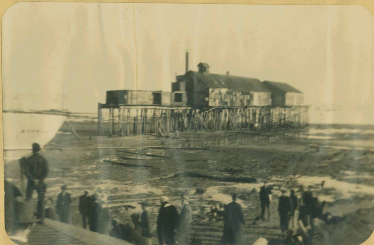
George O. Knowles Wharf after the cutter Morrill and the storm of November 16, 1926 got through with it. Clipping, above picture and pictures on next page given to Althea by Lizzie Livingston.
