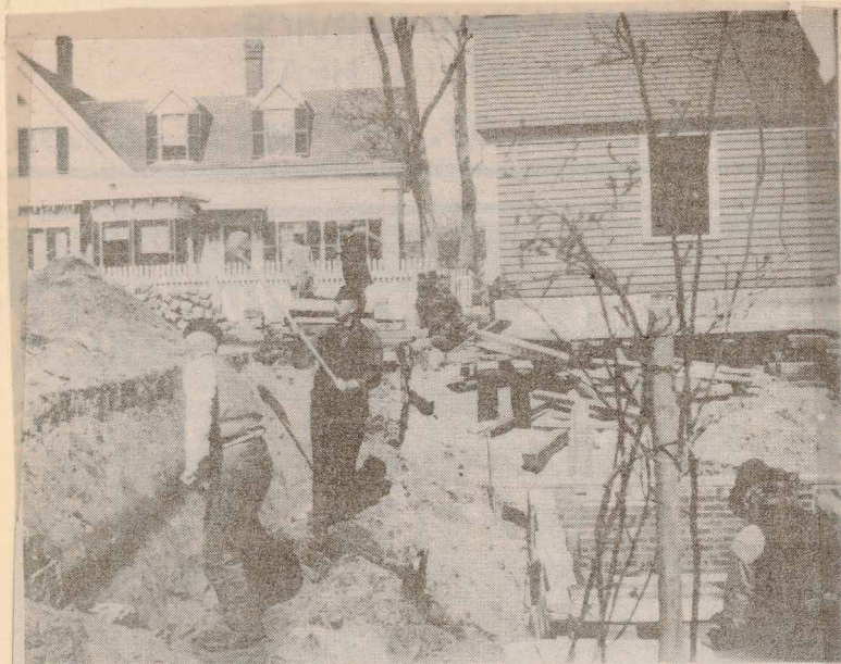
Lower Cape Codders were quite skilled in moving heavy objects. Various "lever and screw" companies operated here in the 19th Century. Usually practice was gained salvaging the hulls of ships on the outer shores, often during unpleasant weather. Above, about 1900, on Tremont Street a store was moved and turned 90 degrees before being attached to a house which fronts on Mechanic Street.
