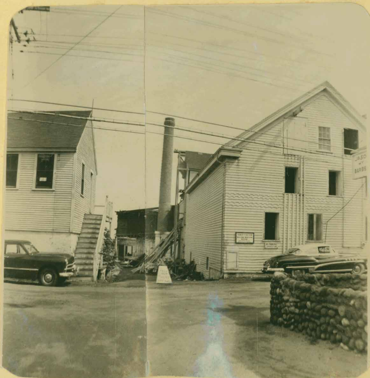
... ..Provincetown Cold Storage, being torn down - May 1952. This is opposite Johnson Street.
