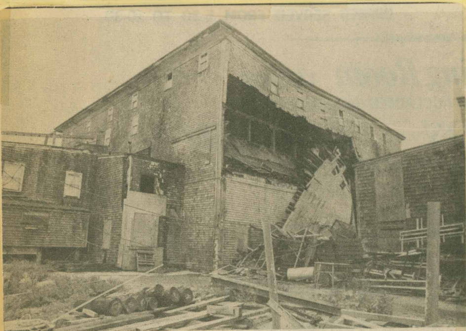
Innards of abandoned Cape Cod Storage plant see light of day where east wall fell from top three floors Sunday. Roof sags over 40-foot opening.
