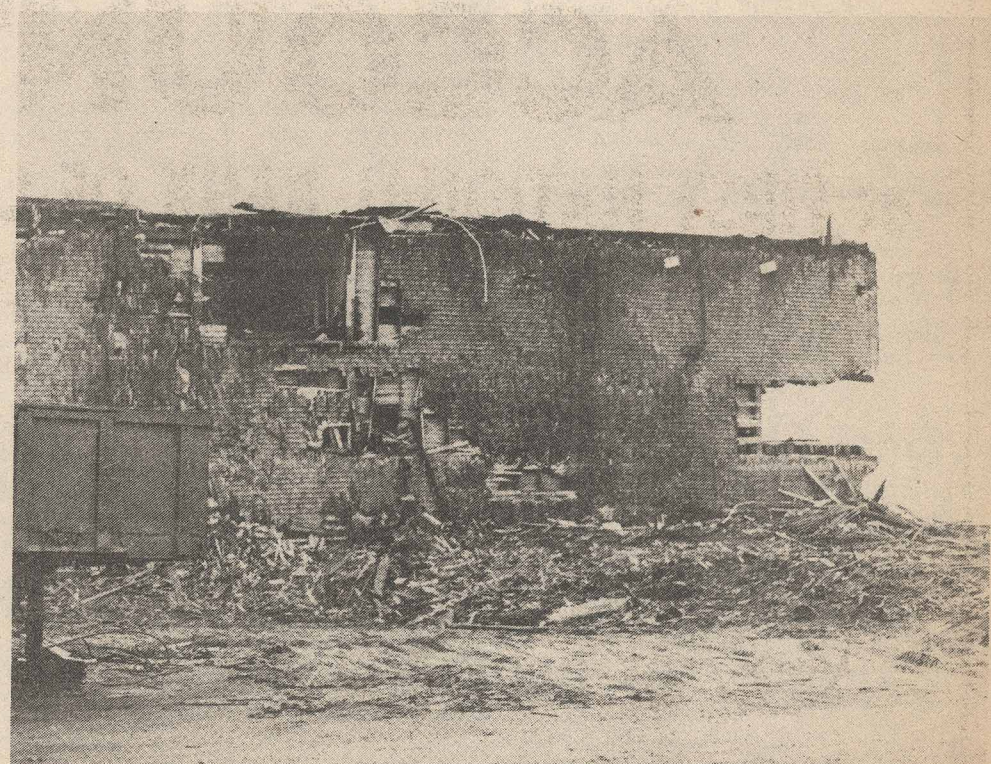
Looking like a beached whale yesterday, the Cold Storage Plant bleakly awaits its final destruction.
